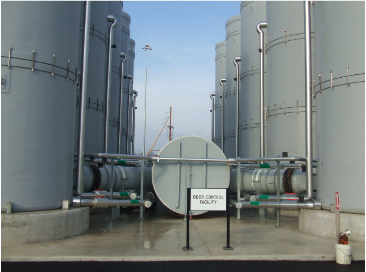
Figure 4 – Bio-trickling Filter Units and Inlet Ducting
