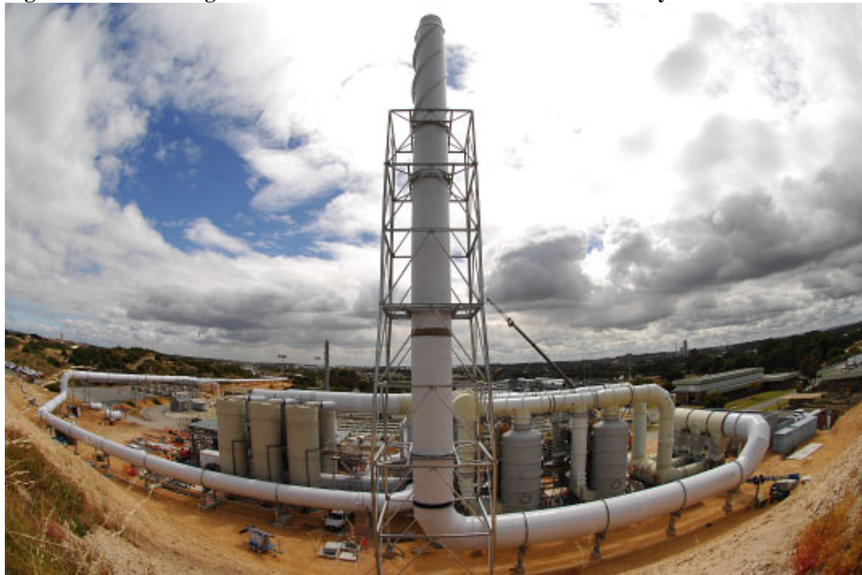
Figure 4 - Biotrickling Filter and Chemical Scrubber Odor Control System with 50m Stack
